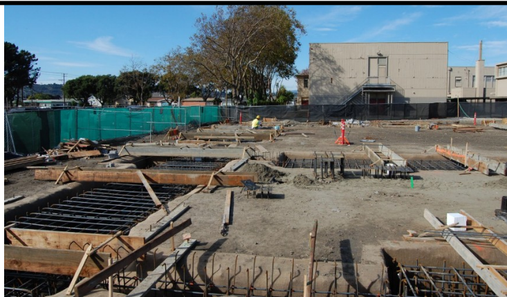
Foundation work for the new Nystrom Elementary School began in 2010 using Measure J bond funds.
